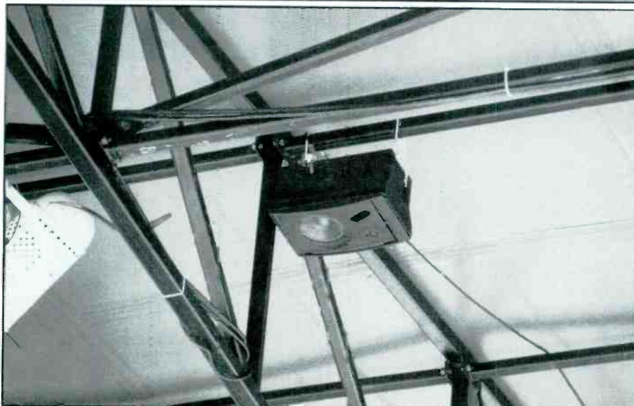
Figure 10. A JBL Control 5 suspended from the reviewing stand's roof.
