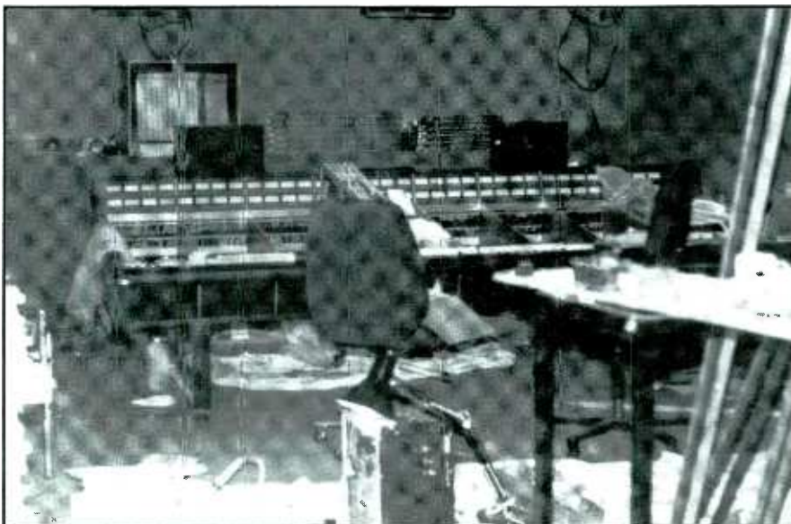
Figure 4. Upon completion, the control room is 15 feet by 27 feet with an annex for meetings. Both are lit with natural daylight.
